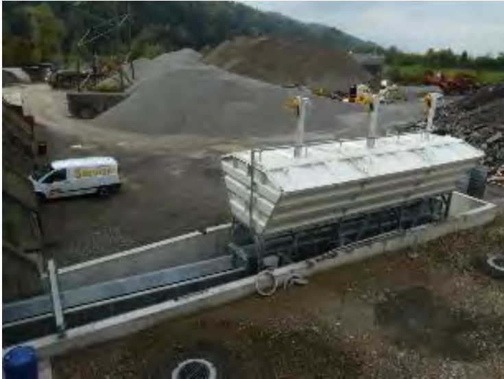
Anlage in Uznach
